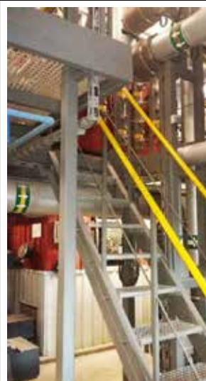
Picture 2. Boiler. (Photo: Vidmantas Verbyla)
