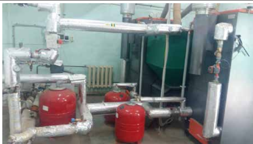
Picture 5. Boiler. (Photo: Valda Gudynaitė–Franckevičienė)
